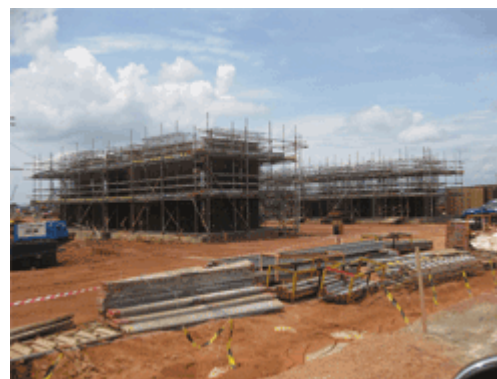
Lynas Corp.'s REE processing plant under construction in Malaysia, which has encountered some local opposition to the
