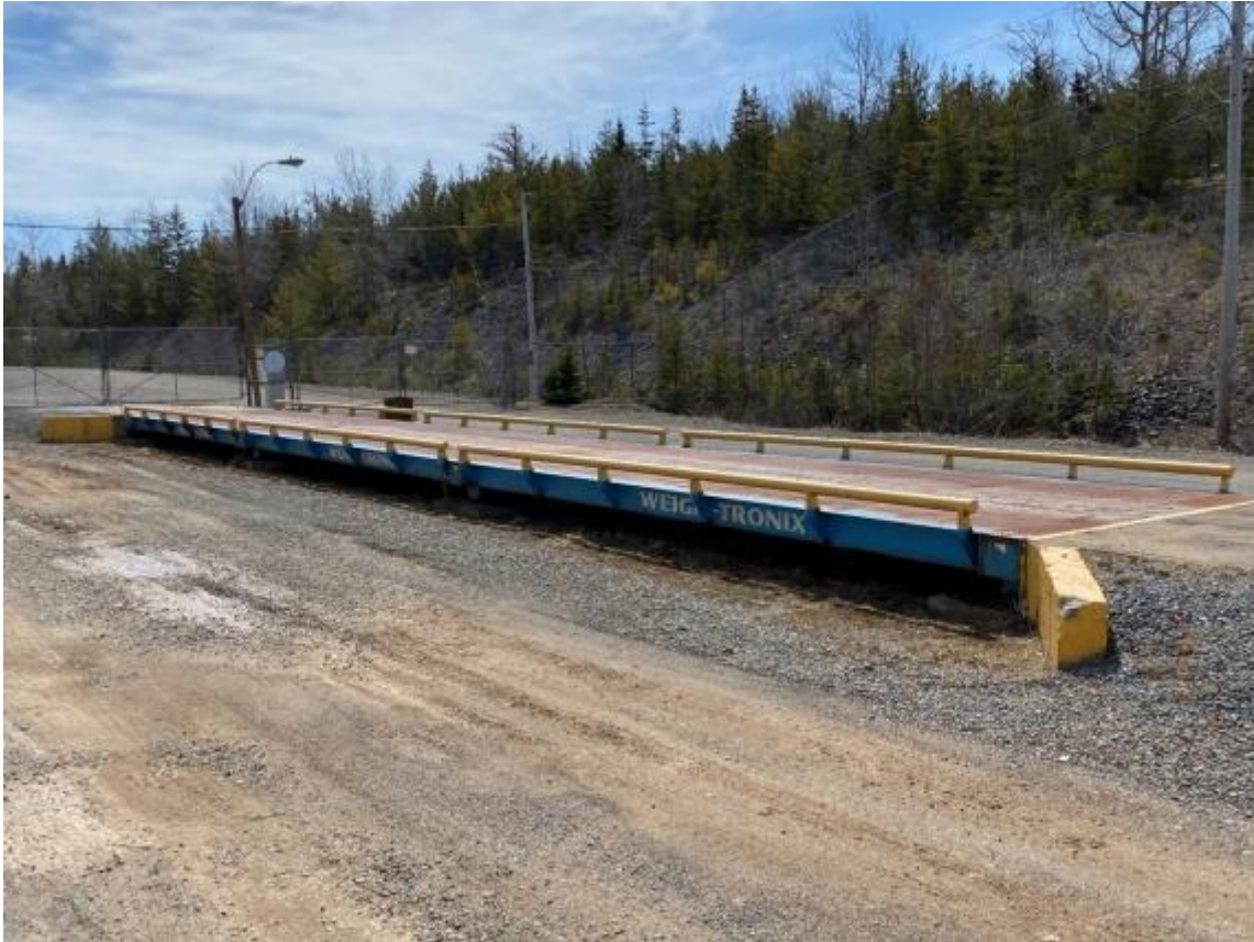
Figure 18-73: Onsite container weighbridge
