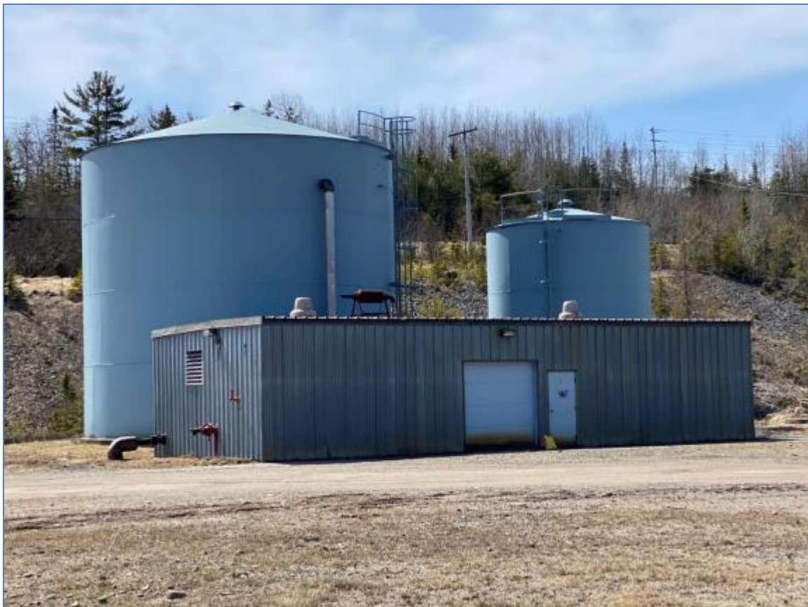
Figure 18-7: Water treatment plant and water storage
